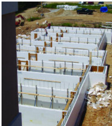
[Top] Insulating concrete forms are stacked like blocks and filled with reinforced concrete. PHOTO COURTESY OF TEAM OXYGEN, SALT LAKE CITY
